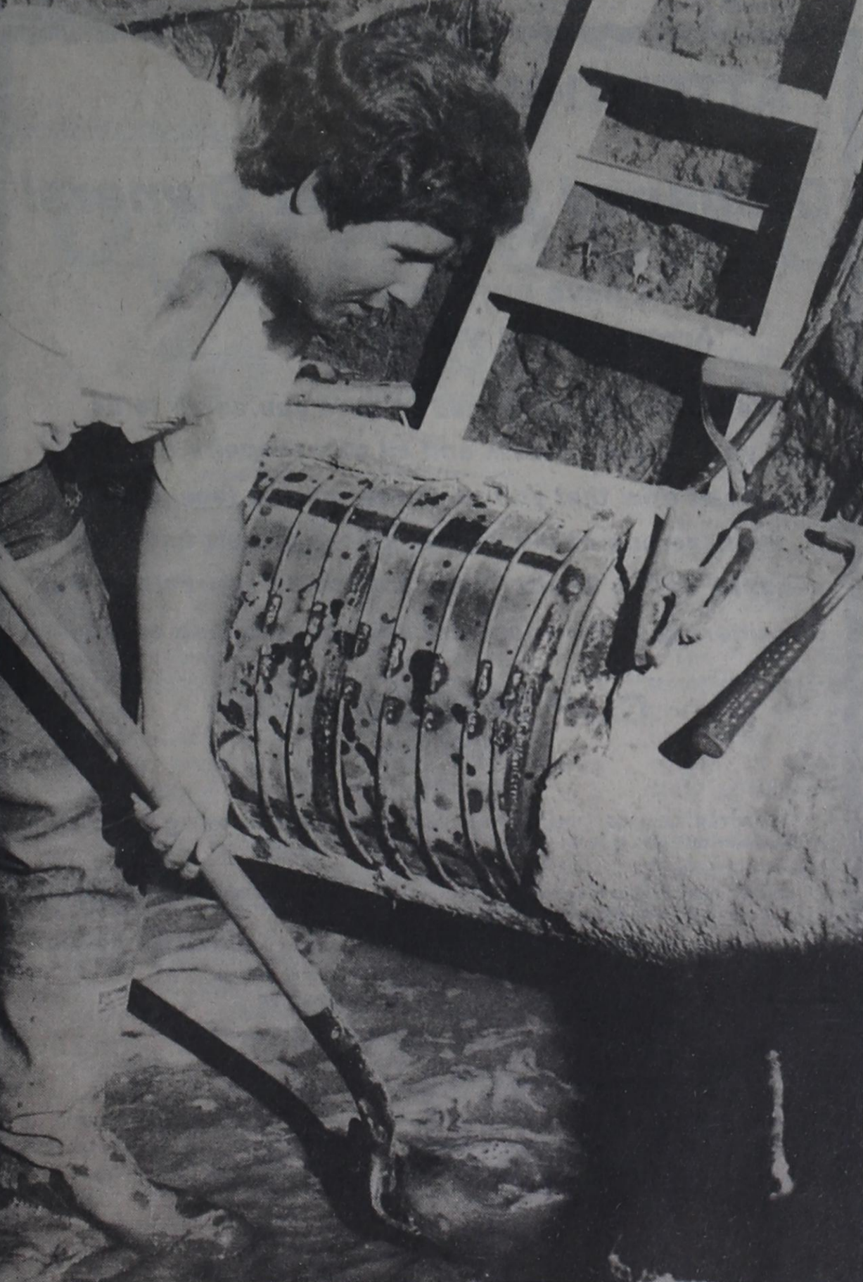
WATER MAIN LINE BREAK - The main water line between Post and White River sprung a leak last week, rusting through from the inside. White River employee Todd Davis begins the cleanup following repairs to the line.
