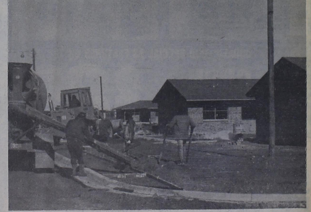
HOUSING PROJECT - Construction work on the new city housing project is taking shape, and with a little sunshine Hoover Construction Company crews began pouring concrete this week. When completed, there will be a total of 30, one bedroom units, with three specifically built for handicapped. The units will be available to people 62 years or older and those who are physically handicapped. Details about the housing project may be obtained by calling 495-2233.
