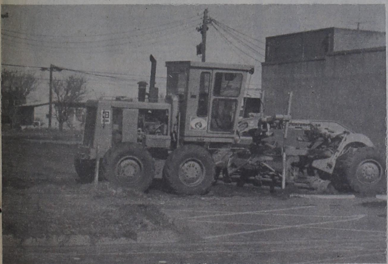
DOWNTOWN PARKING LOT - Work is proceeding on the Post Merchants Association's sponsored downtown parking lots, as city crews prepare the lot on East Main Street. Plans call for city crews to prepare the lots in conjunction with other street maintenance projects.
