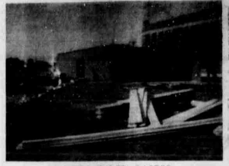
WORK GOES FASTER Improved weather conditions have brought a resumption of work on the new law enforcement complex and jail being built on the west side of the courthouse. Workmen expect to put the roof on the new building in May.—(Staff Photo)
