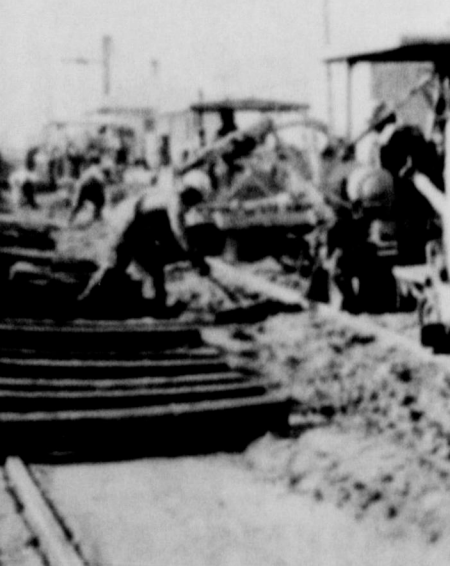
WORKING ON DE RAILROAD—These three pieces of equipment were "ground" near the Knox City Santa Fe Depot Wednesday morning as crews replaced of cross ties. The first machine pictured right, was sawing the old and lifting them out to the side of the tracks. The second machine inserted and lifting the third machine held the new ones in place and spiked them. Foreman J. I. Smith, local agent, said that any person who had any of the old cross-ties was welcome to them—to just come "haul them
