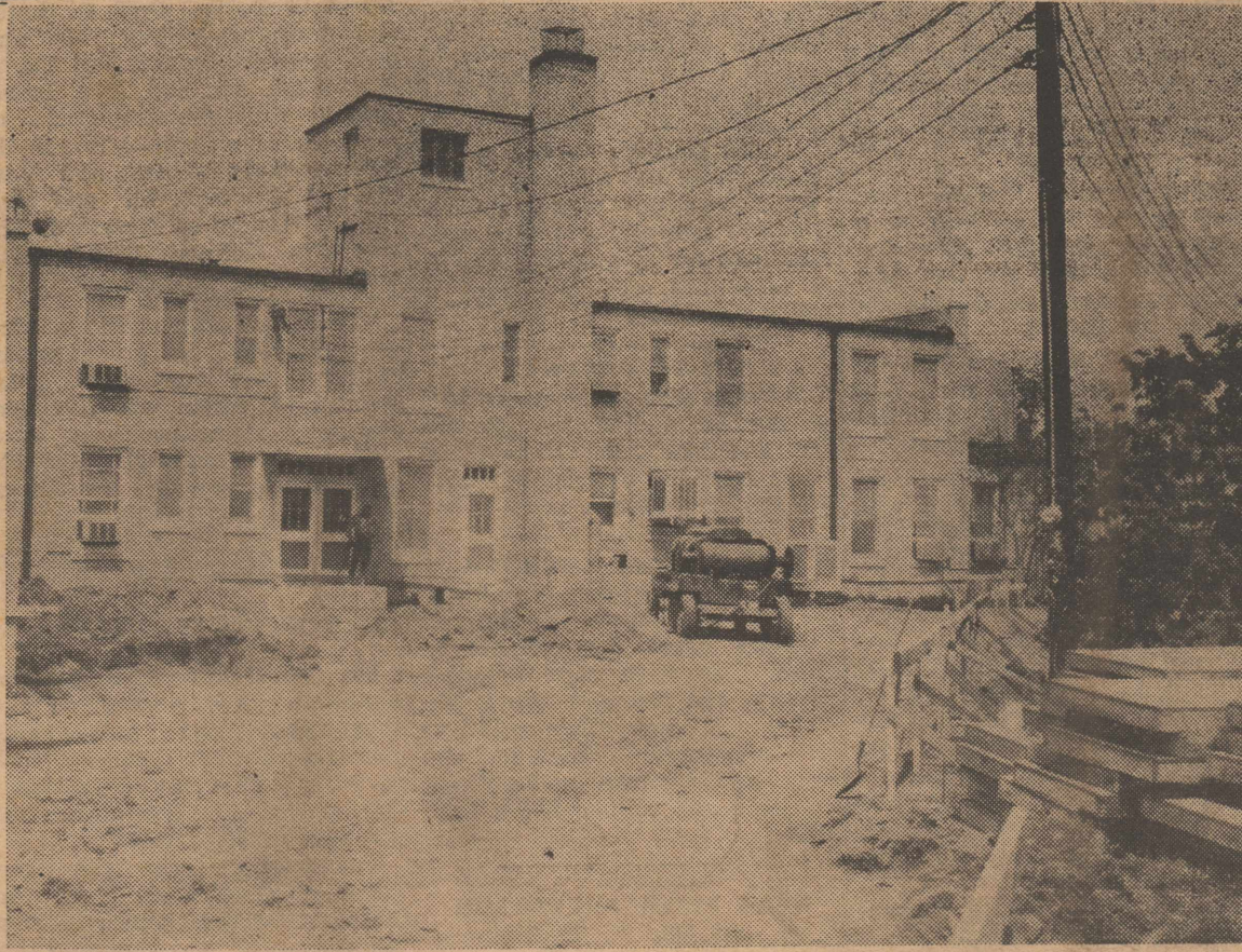
WORK BEGINS — Shown above is the south side of the Knox County Hospital where work began last week to add additional rooms and renovate the existing structure. Work also started on the Courthouse and contractor for the buildings is T. E. Shelburne & Son, Inc., of Snyder. They submitted the low bid of $157,478 for both buildings.
