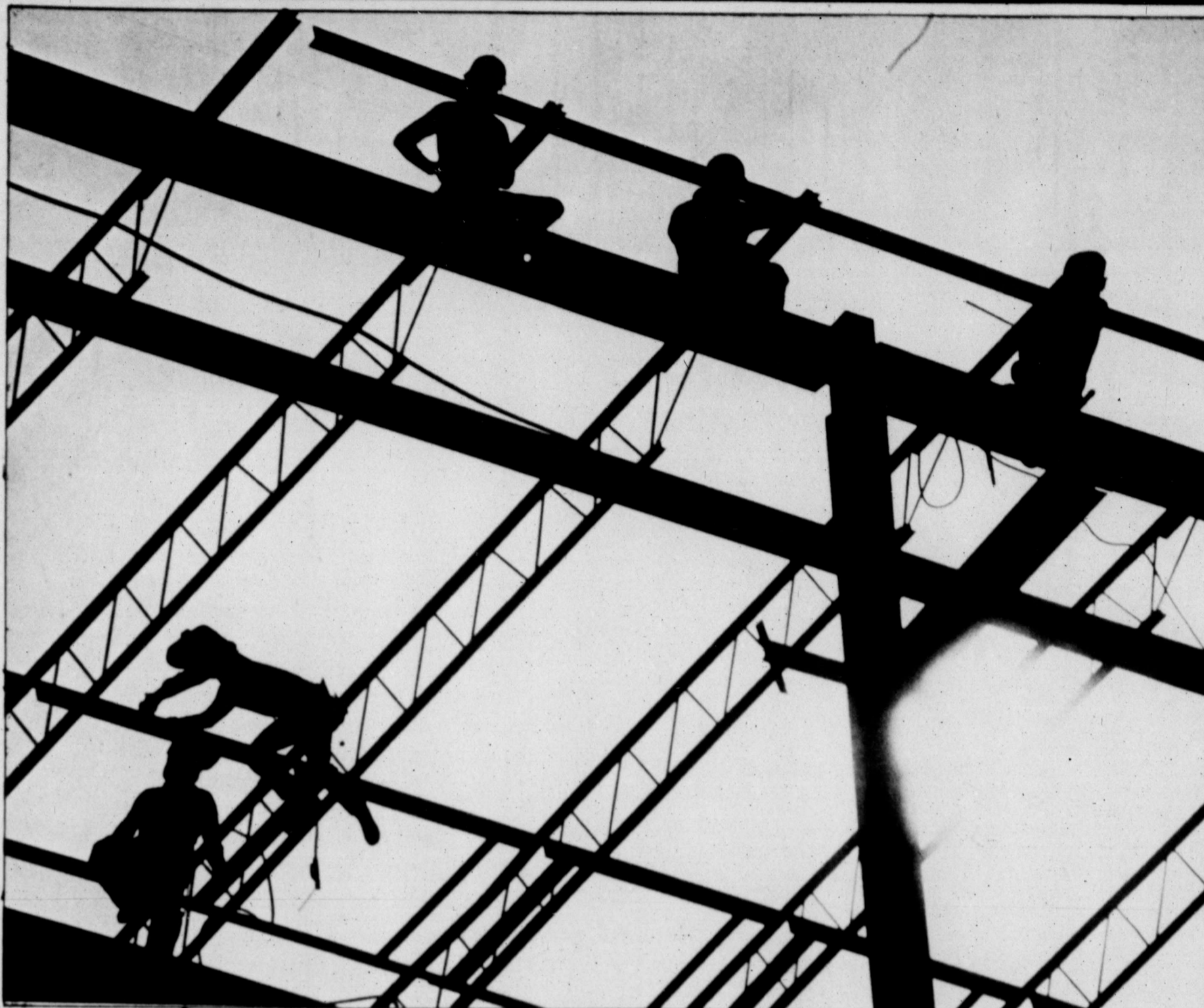
A warm January sun silhouettes welders atop the Paragon building near downtown Midland Wednesday. The Paragon, an 11-story, $18 million building located at Marientfeld Street and Louisiana Avenue, is one of several major office complexes now under construction in Midland. (Staff Photo by Paul Gilbert)
