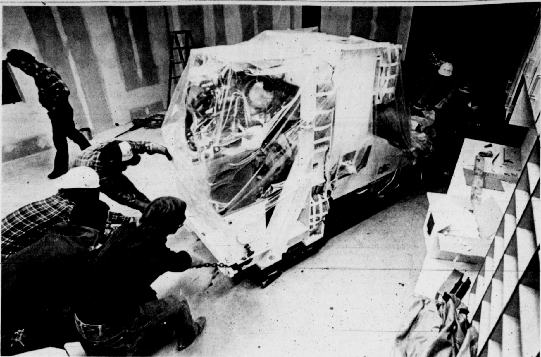
Workmen from Area Builders Inc. give it the "old heave-ho" as installation begins on the Allison Permian Basin Cancer Therapy Center's 20 Million Electron Volt linear accelerator Wednesday. Part of a wall had to be removed Wednesday to fit the monster machine into its special room. The 6 MEV is scheduled to arrive today.
