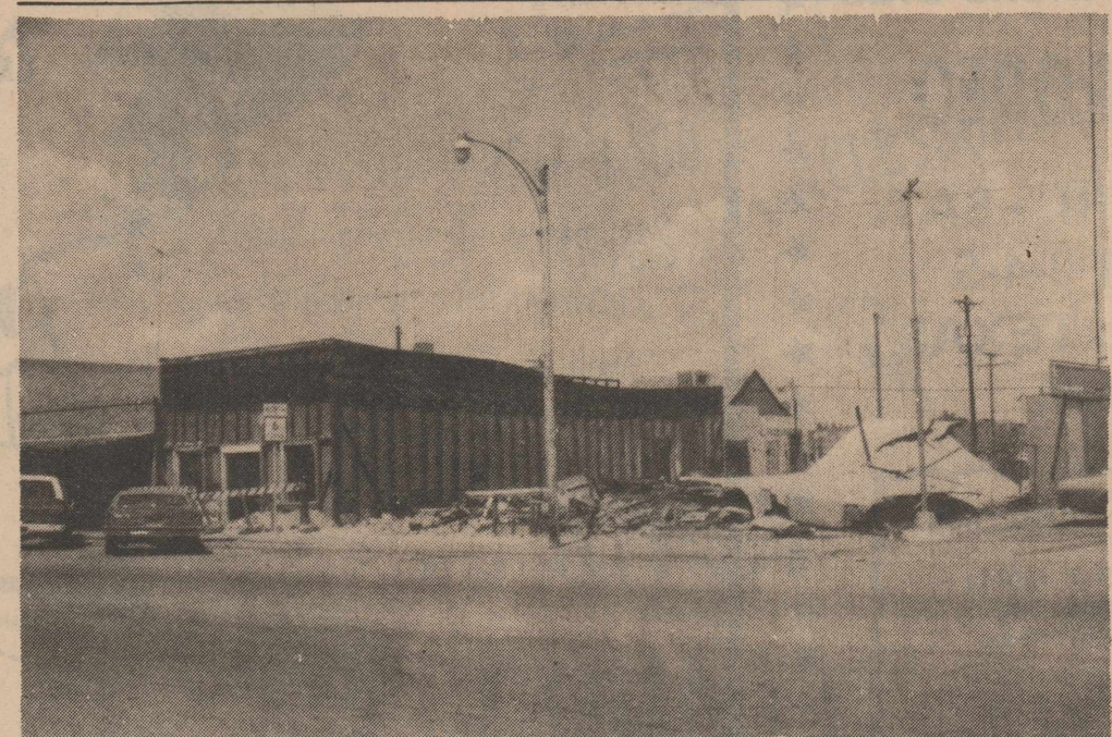
ALTHOUGH THIS MIGHT LOOK LIKE the aftermath of a storm, actually these buildings on Central Avenue north of the Mobil Station are being torn down to make room for additional parking and a mini-park to beautify the downtown business district. Several months ago the Knox City Chamber of Commerce took the improvement as a project with businessman David Counts as the Chamber official in charge. Counts said that plans call for the area to be leveled with 10 or 15 feet of the front area being set aside for the mini-park with several shade trees and park type benches. The area near the street will be sealed off and access to the parking will come from the back, Counts said.
