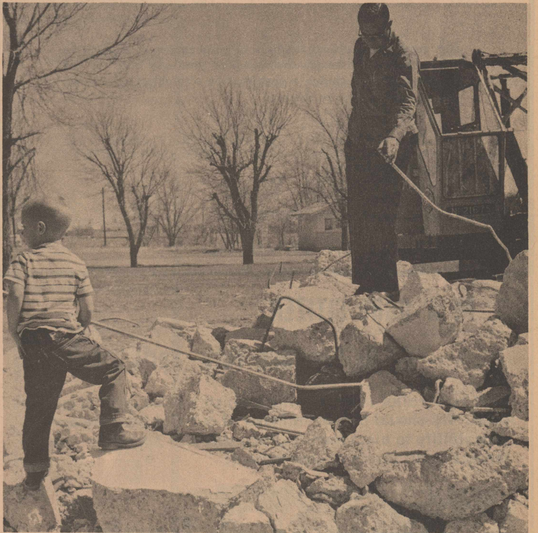
CHIP OFF THE OLD BLOCK—Like his dad, Scott Fite, 4, son of Dr. and Mrs. Lynn Fite, is interested in the progress being made by workers who have been breaking up concrete on the square. The concrete was the basement of the old hospital. By Wednesday, workers had most of the concrete out. They used a 1700-pound ball to break it up. The concrete was the last obstacle to getting the square cleaned up.
