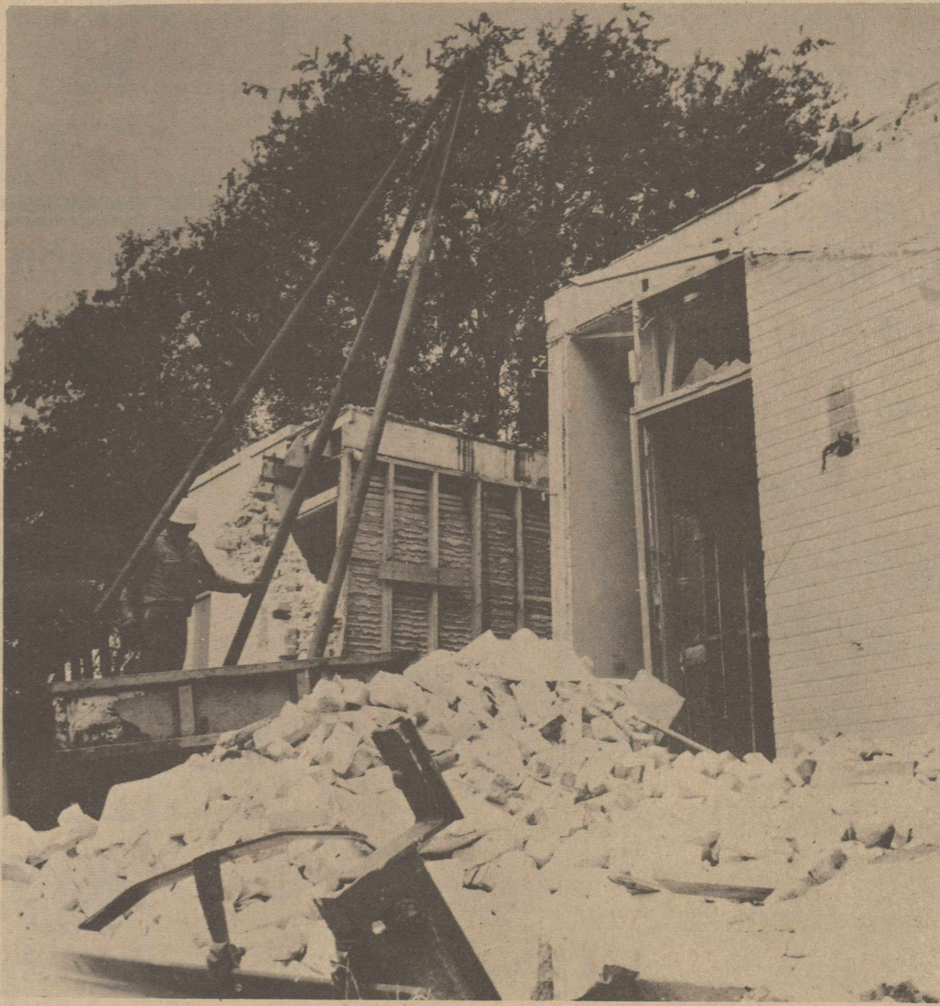
HOSPITAL TURNS TO RUBBISH---This shows the south side of the old hospital building, after workers pulled all the walls of the second story and began razing the bottom floor. Here a workman is shown clearing the old elevator shaft of the hospital. Demolition is expected to take about three more weeks.
