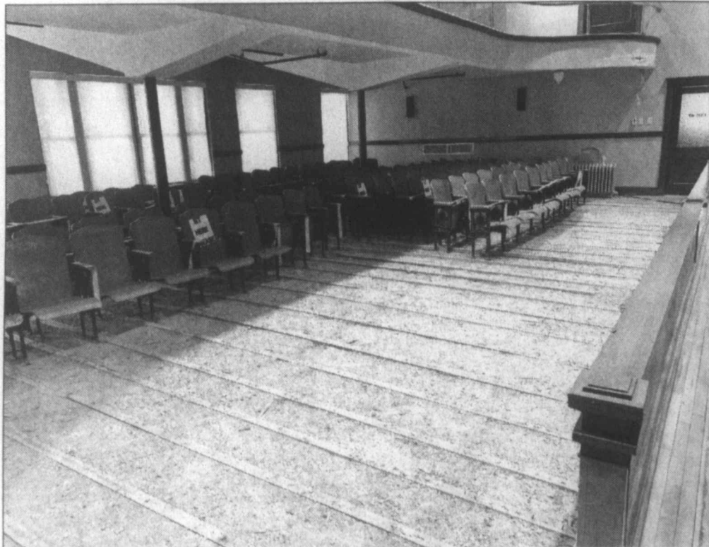
No floors in district courtroom ... The maple wood floors were pulled up in the District Courtroom on the second floor of the Lynn County Courthouse, after a major flooding incident occurred last May, and the courtroom has been unused since then. Repair work is set to begin soon. (LCN PHOTO by Juanell Jones)
