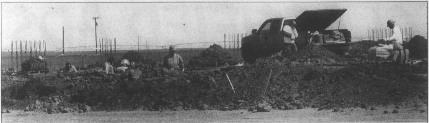
Dirt work ... Dirt work continues at the Tahoka ISD site for the new gymnasium, field house, baseball and softball complex on N. 5th Street in Tahoka. The project is funded with a bond that voters approved last year. (LCN PHOTO by Juanell Jones)
