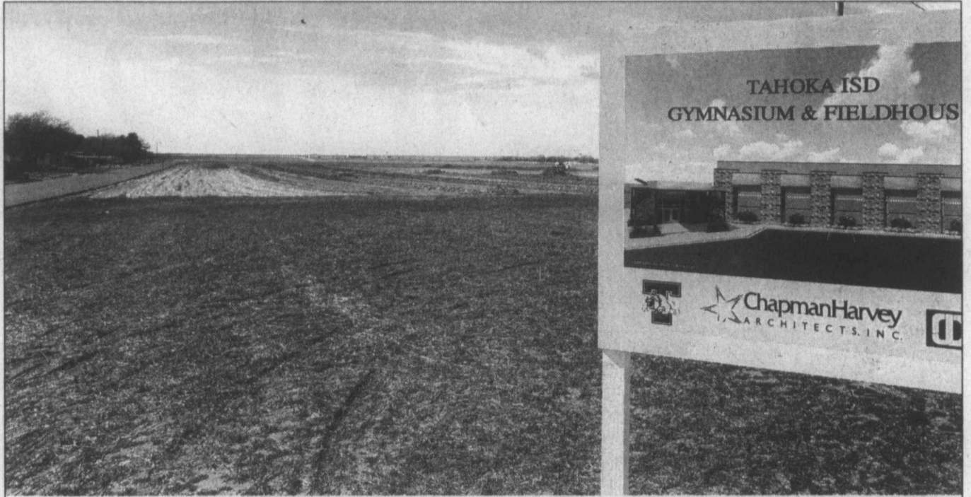
Groundwork begins ... Groundwork began last week on the Tahoka ISD bond project, on land bordered on the south side by North 5th Street, and on the east side by Avenue P. A new gymnasium, field house, football practice field, and baseball and softball field complex is being built here. It is anticipated that the new gym and field house will be completed by December 2020, and that the baseball field and softball field will be completed before the 2021 spring sports season. The football practice field will need time for the grass to root so it will most likely be another year before the practice field is used.
