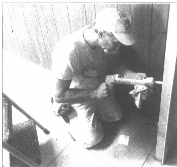
Preparing to paint ... Gary Martindale prepares the walls for painting at the former Tahoka City Hall on Lockwood Street, which will soon be the new location for the Lynn County Pioneers Senior Citizens Center. The smaller offices will be used as classrooms or for other activities at the new center.
