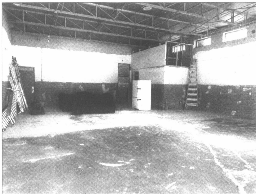
Transformations underway ... This area, formerly the garage/fire truck area at the former Tahoka City Hall on Lockwood Street, is being transformed into the dining area for the new Lynn County Pioneers Senior Citizens Center. New concrete has been poured to raise the floor, which will be tiled, dropped ceilings/insulation will be added, and walls will receive a new coat of paint. New windows and front entry doors will replace the garage doors.
