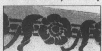
Gold leaf on walls ... This is an up-close look at the gold leaf pattern that has been restored near the ceilings of the District Courtroom in the Lynn County Courthouse restoration project. (LCN PHOTO)
