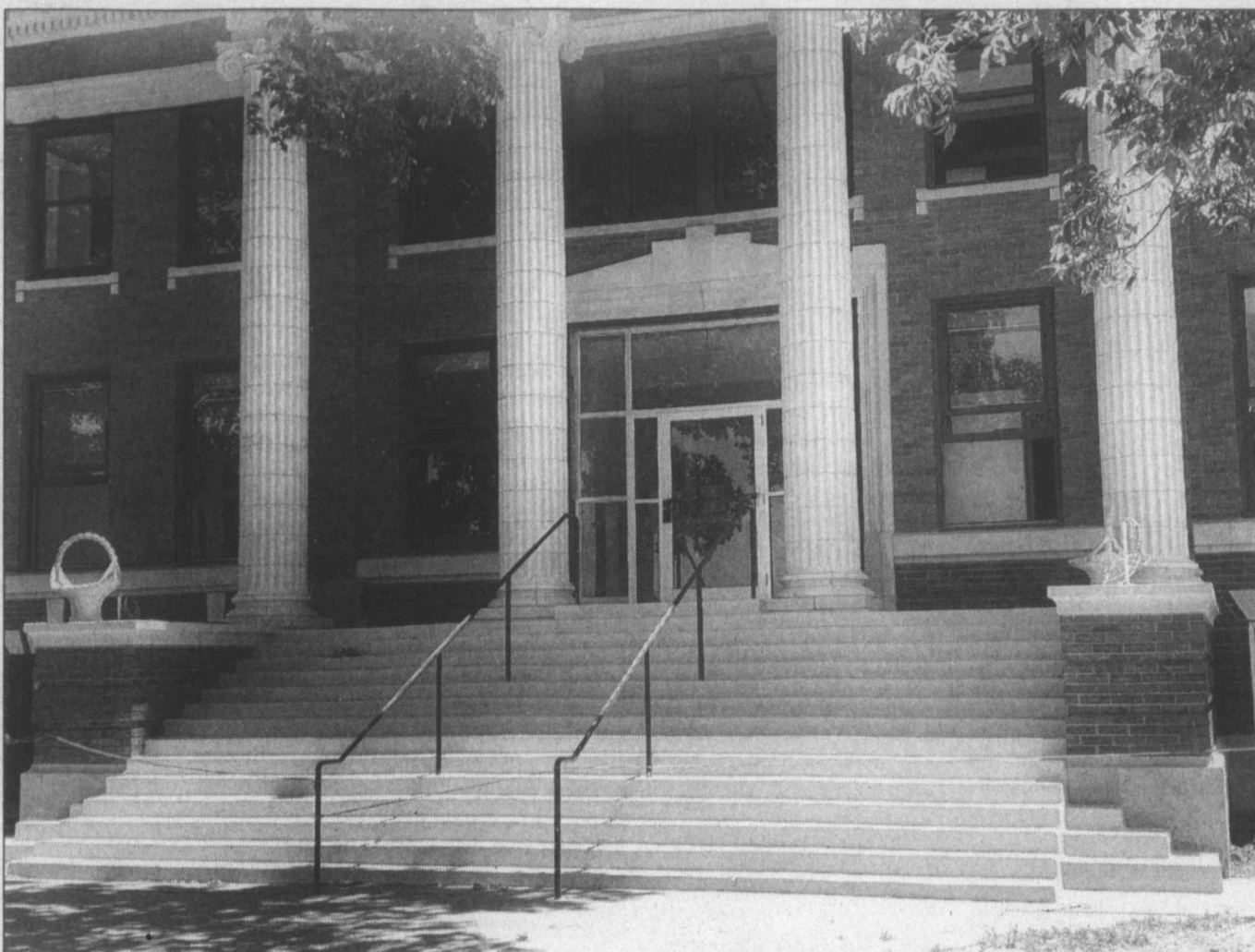
Updated steps ... The concrete steps leading to the Lynn County Courthouse have received an update, covering the cracked concrete with a new finish that improves not only the looks of the steps but the safety as well, with a fine-sand non-skid finish. Restoration of the courthouse is expected to be completed soon, with a grand opening/rededication slated for July 20.
