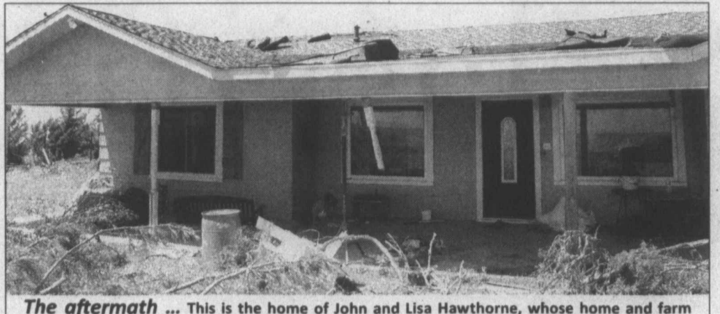
The aftermath ... This is the home of John and Lisa Hawthorne, whose home and farm and suffered damage after a tornado whipped through Sunday evening, near Draw. Front porch posts were ripped from beneath the front porch, and on the back side of the house, the roof was peeled off and a ceiling collapsed inside a bedroom. No one was home at the time. (LCN PHOTO by Gary Jones)
