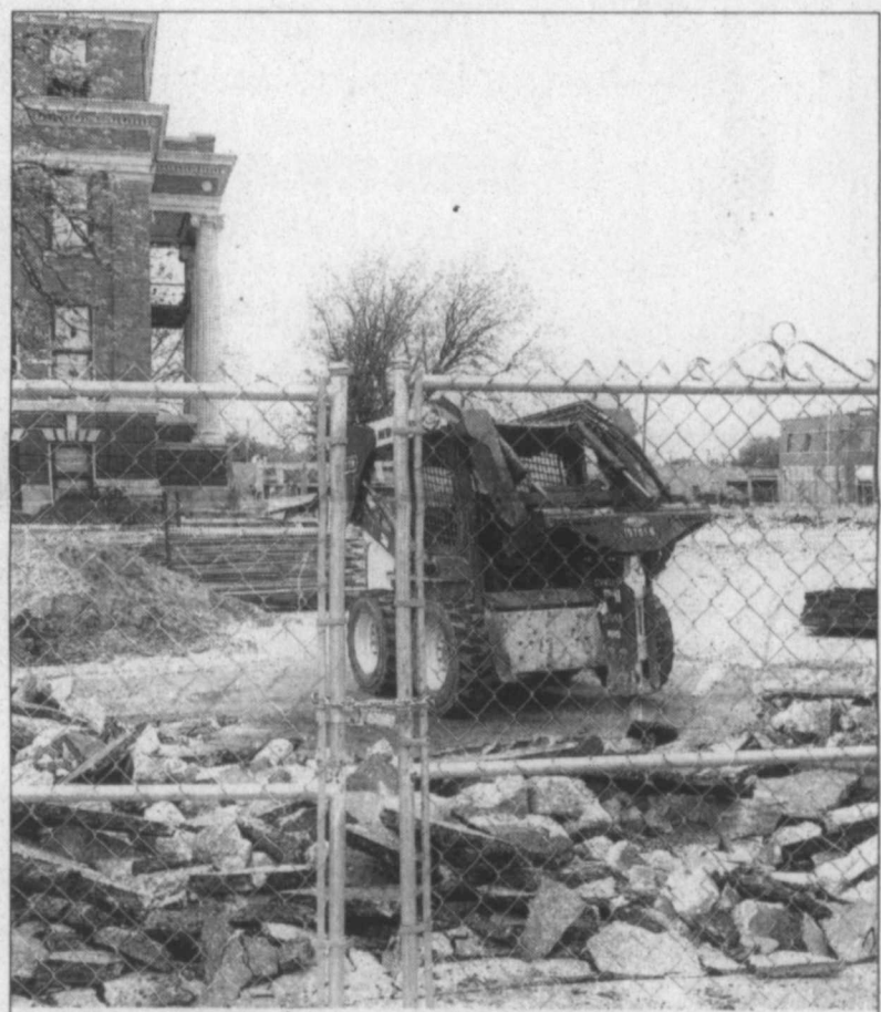
Street removal ... The street that curves from Main to Ave. J just west of the Lynn County Courthouse is being removed, and will become lawn area for the courthouse, returning the downtown area to a true square. It's part of the courthouse restoration project that is expected to be completed by this summer. (LCN PHOTO by Juanell Jones)
