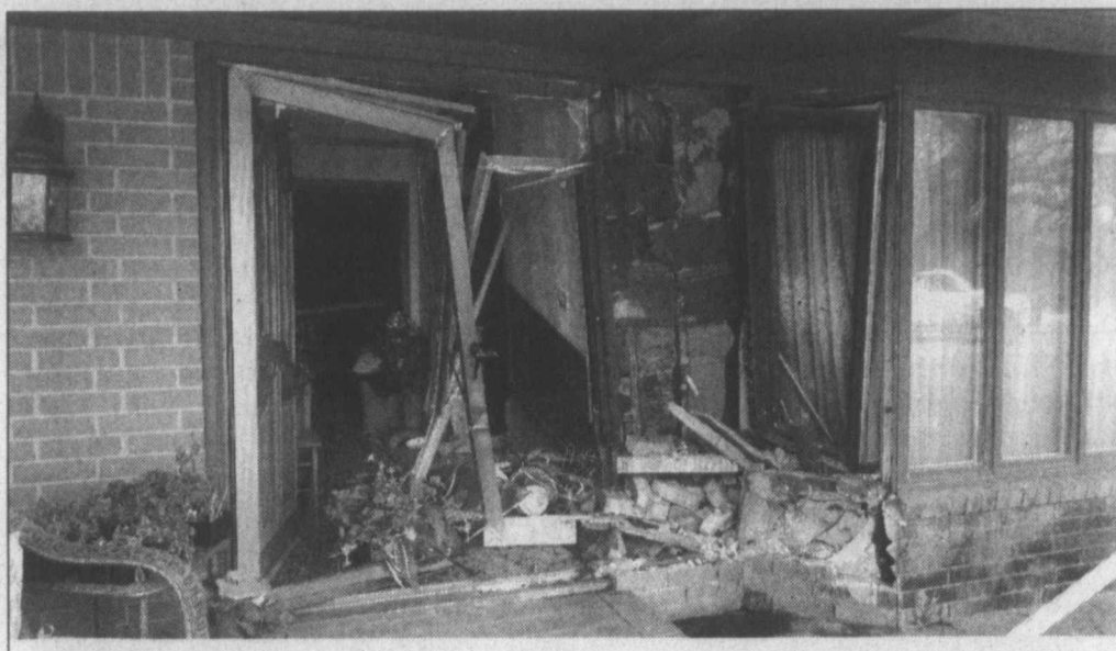
Accidental impact ... After backing up to her front porch to unload flowers, Vickie Dunn accidentally hit the gas while in reverse in her Ford Explorer, crashing through the front of her house in the 1700 block of N. 7th, damaging both her vehicle and her home last Friday. Tahoka Police responded to the scene, and an officer stayed until the home was secured.
