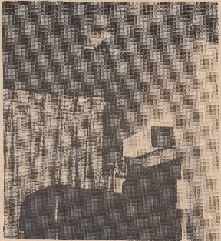
SOP IT UP —Late at night west third floor residents were rudely awakened when water poured out of the ceiling. Repairs are not planned until spring break according to David Harr, residence hall director. See story page 1. —Jana Harris photo
