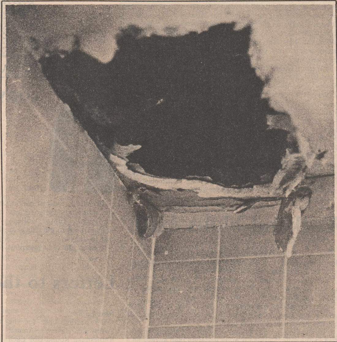
THE BLACK HOLE—Pipes bursting in the dorm caused heavy damage to this shower on North-1st. —Kevin Starnes photo
