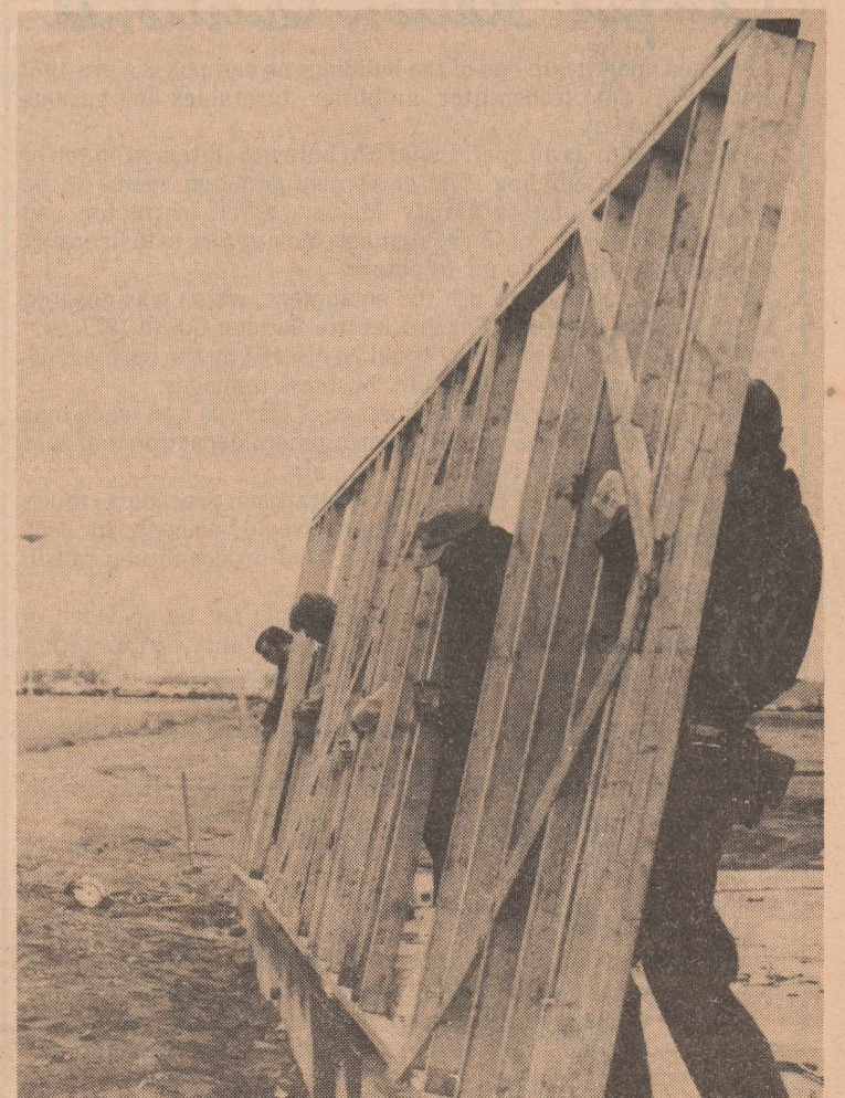
WALL-TO-WALL — Residential construction students Kenneth Baker, Sammy Simmons, Phil Jones and Maury Moore stand a wall on the second duplex. (photo by Lois Gleason)
