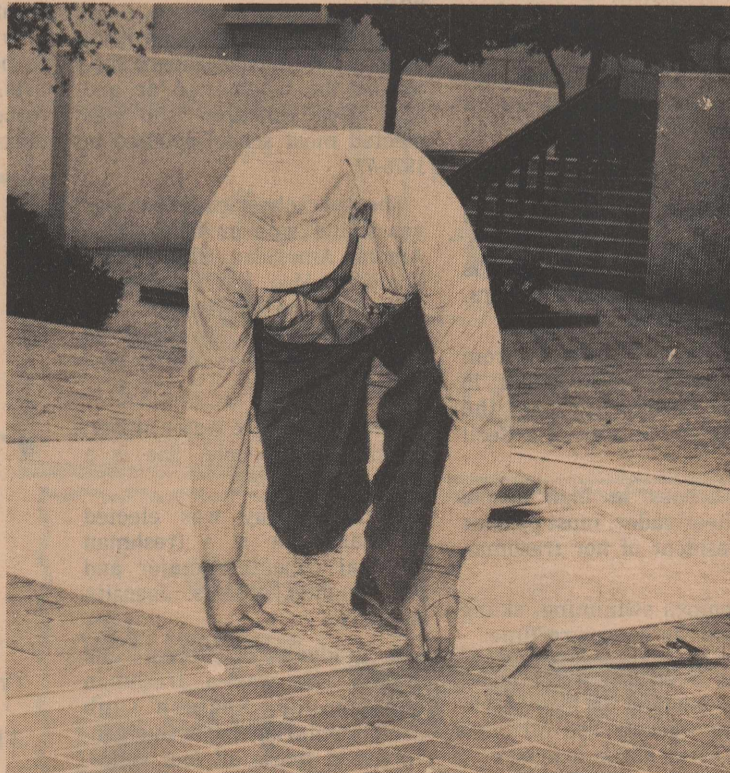
HARD AT IT — George Light, maintenance repairman, puts trim around the platform in the courtyard. (photo by Joe Boldon)
