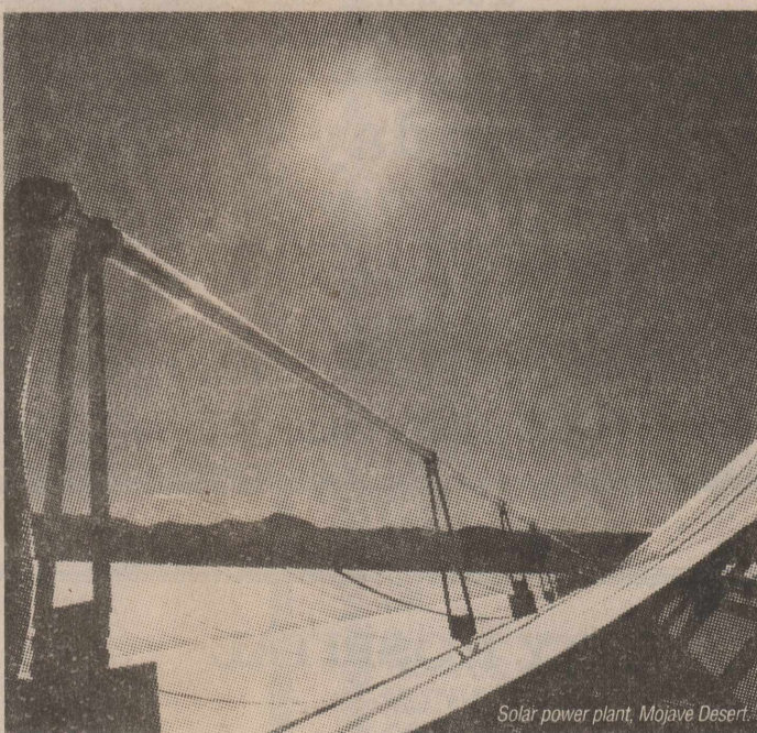
Solar power plant, Mojave Desert.
