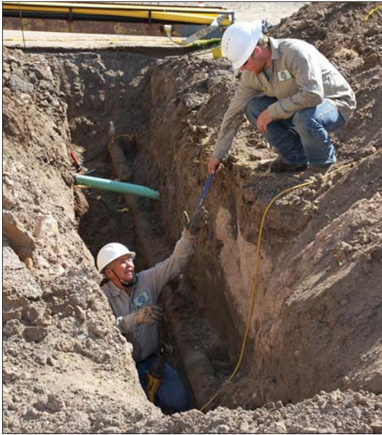
Gas work GreenLight Gas employee Chase Galyean hands Keith Troser a new blade as they work to cut through the old gas pipe behind the businesses in the 100 block of S. Kearney Street Tuesday. The crew is hoping to have the job finished in the area after Thursday.
