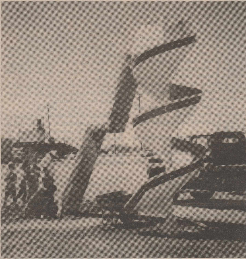
Mike Juarez and Mark Eddleman have been completing the installation of a new slide on the Silverton Elementary School playground this week. Several weeks ago a new merry-go-round was installed, and both pieces of play equipment were purchased with school funds earmarked for that purpose. Briscoe County News Photo
