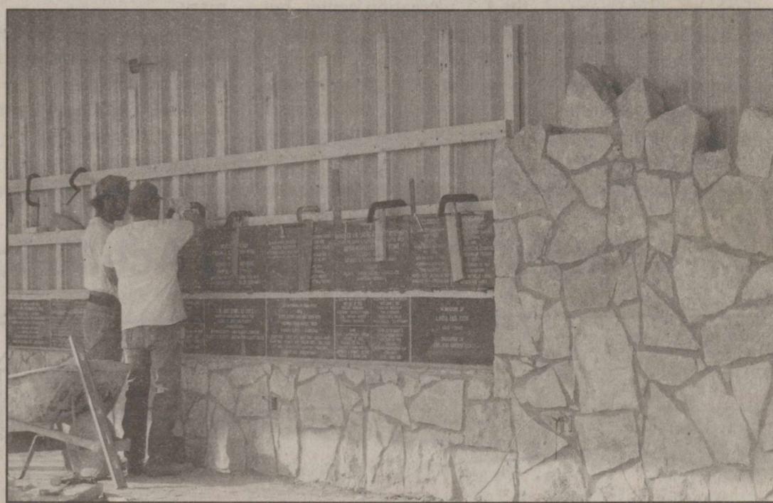
Dale Huffman and Kevin Urbanczyk began placing the granite plaques on the museum facade this week. Progress on the exterior is rapidly being made
