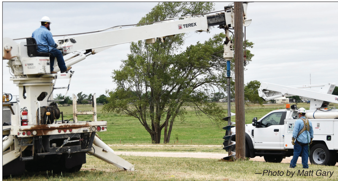
LABOR AND EQUIPMENT DONATED: Greenbelt Electric Coop workers pull old light poles to make way for dirt work to rework baseball fields at Tom Britt Memorial Park Wednesday, May 20, 2020.
