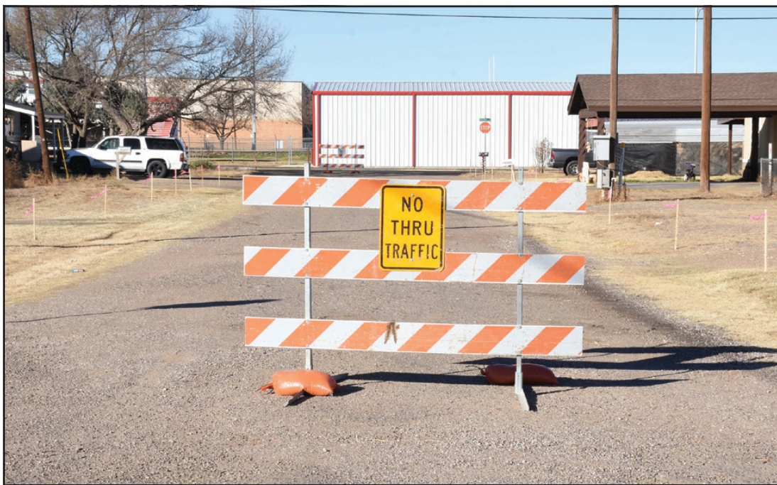
Word on the street — work is underway to finish 8th Street between Ashland and Grand. Paving and curbing will be installed. This work is part of the Friona City Council’s goal to finish unpaved streets around town in the upcoming years.
