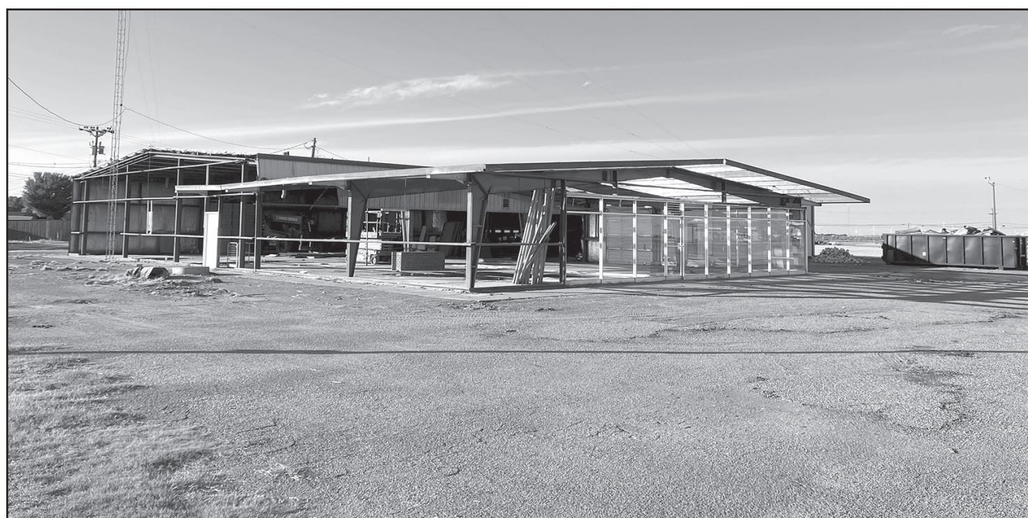
Deconstruction of the old 4-Way Pump building is underway. Plans are underway to repurpose the property with new retail businesses, a business park with office rental, and a food truck park area.
