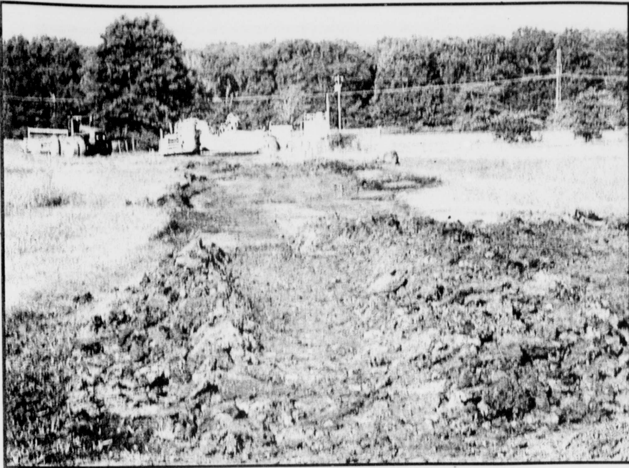
DELAYED-The dirt work which was to have been started at Rivercrest has been rain delayed. Although machinery attempted to begin progress recent rains put a quick halt to the work. (Staff Photo Nancy Brown)
