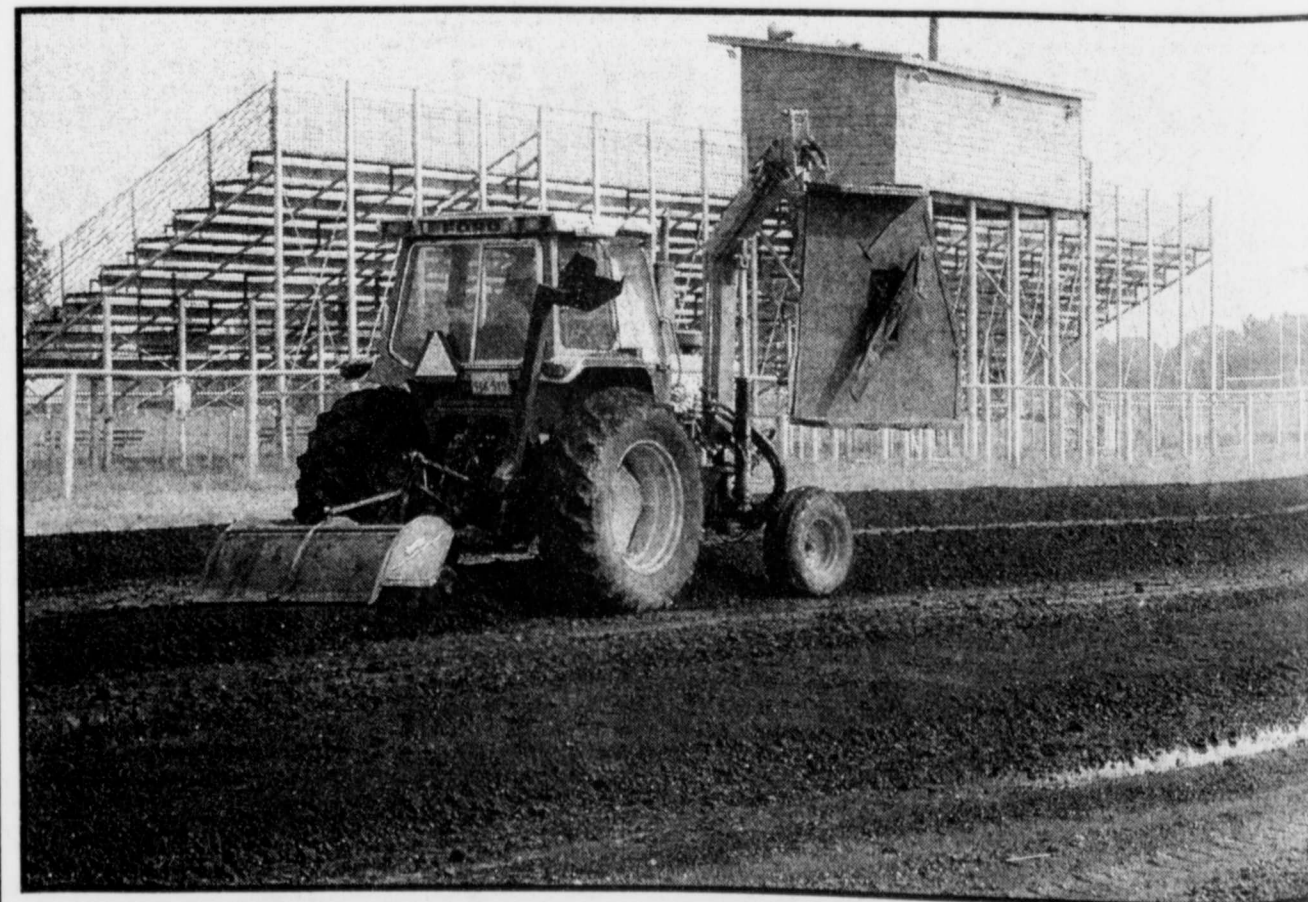
NEW PARKING LOT -The Rivercrest Rebel football parking lot was getting a facelift this past week. Red River County Commissioner, Ricky Daniels and crew were working hard to get the lot repaved before the season gets into full swing. (Staff Photo Nancy Brown)
