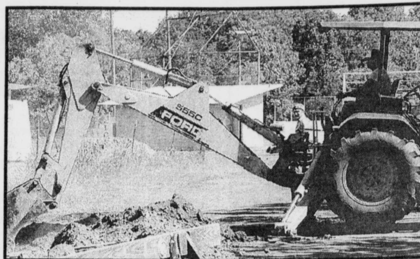
CONSTRUCTION COMPLETE-Talco Ball Field was excited to open their new bathroom facilities this past week. The work was completed on Tuesday. Pictured are city worker Charles Huey and Randy Hollis the Girls Softball Director and Vice President of the league. Staff Photo Nancy Brown
