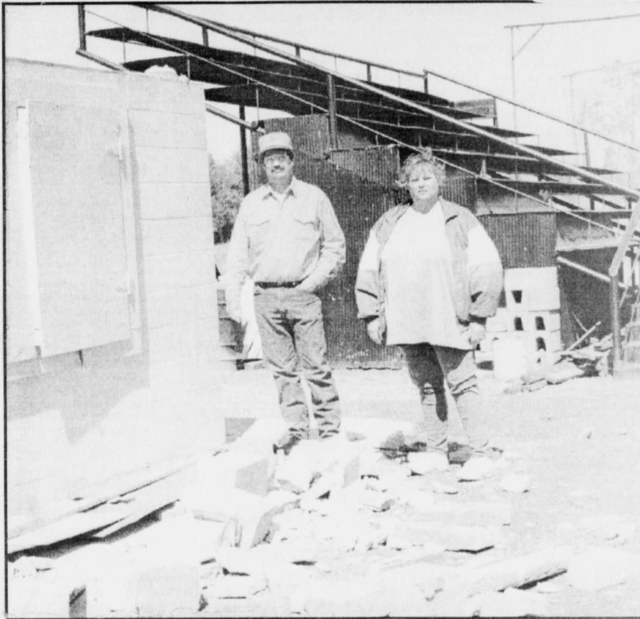
GONE WITH THE WIND -Mark Hare and Rueanna Bell check damage done at the Bogata Ball Park Monday night due to the storm which moved through in the afternoon. The parents just worked to put a new roof and enlarge the building of the concession stand. This depleted the groups funds and damage is estimated at $500. Donations will be appreciated to help repair the damage. The group needs to have the building back in operation as soon as possible since league play began this week. To make donations call: President, Regan Bell-632-5885, Secretary, June Young-632-4863 or Vice President, Mark Hare-632-5150.
