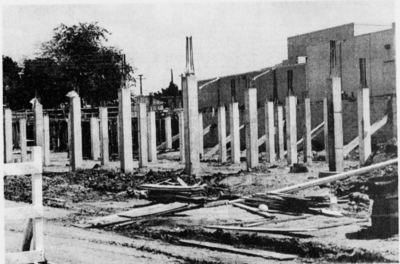
WORK IS MOVING along in spite of the rainy weather on the new jail expansion in Titus
