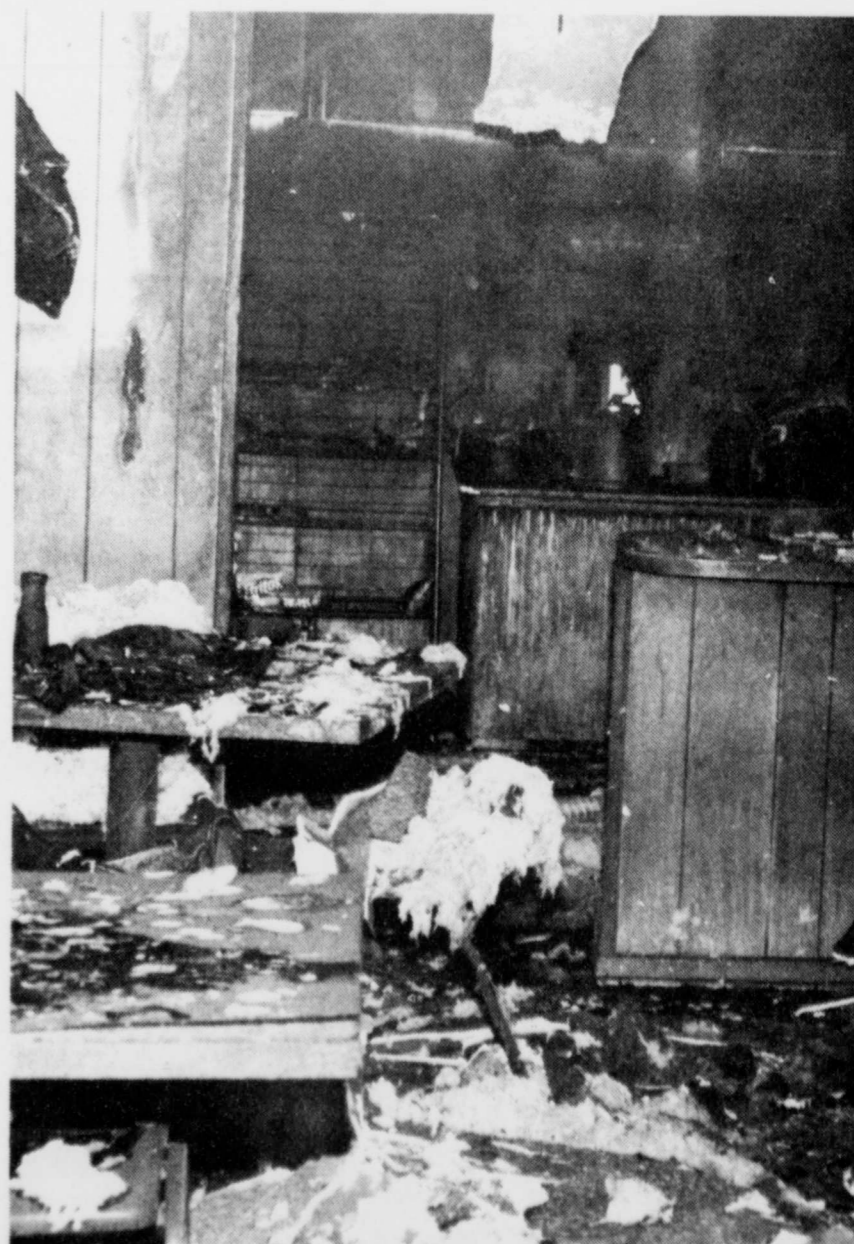
DESTROYED-The Tip Top Cafe in Bogata was completely gutted by fire of an unknown origin Monday night, Nov. 22. The Bogata Volunteer Fire Department responded to the fire, which started sometime after nine p.m. The business was not open at the time. (Staff Photo by Judy Screws)
