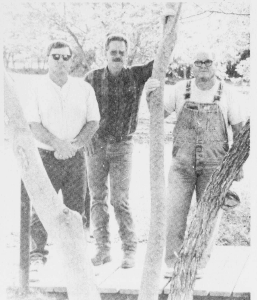
WORK CONTINUES at Talco Park. Saturday saw the completion of the first of three bridges. Ricky Nolen, Bobby Kuhl and Dick Dixon, along with Randy
