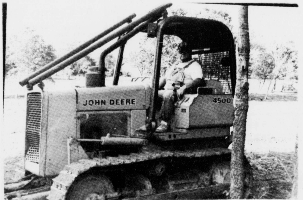
DOZER WORK -Work on Talco Park has continued all last week with the help of J.W. Terrell,
