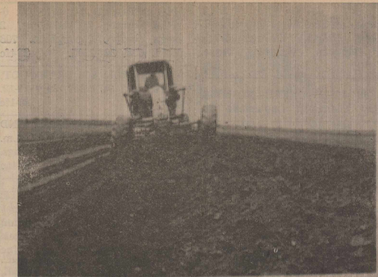
Pictured above is a parallel terrace system being built on the Lem and Max Weaver farm near Brice.
