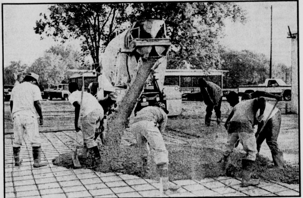
NEW SLAB- Willie - Edward Fulbright and crew were busy early Monday morning pouring the concrete slab for the new bays on the Deport Volunteer Fire Department's station. The new edition should be completed by January 2000. (Staff Photo by Thomas Nichols)
