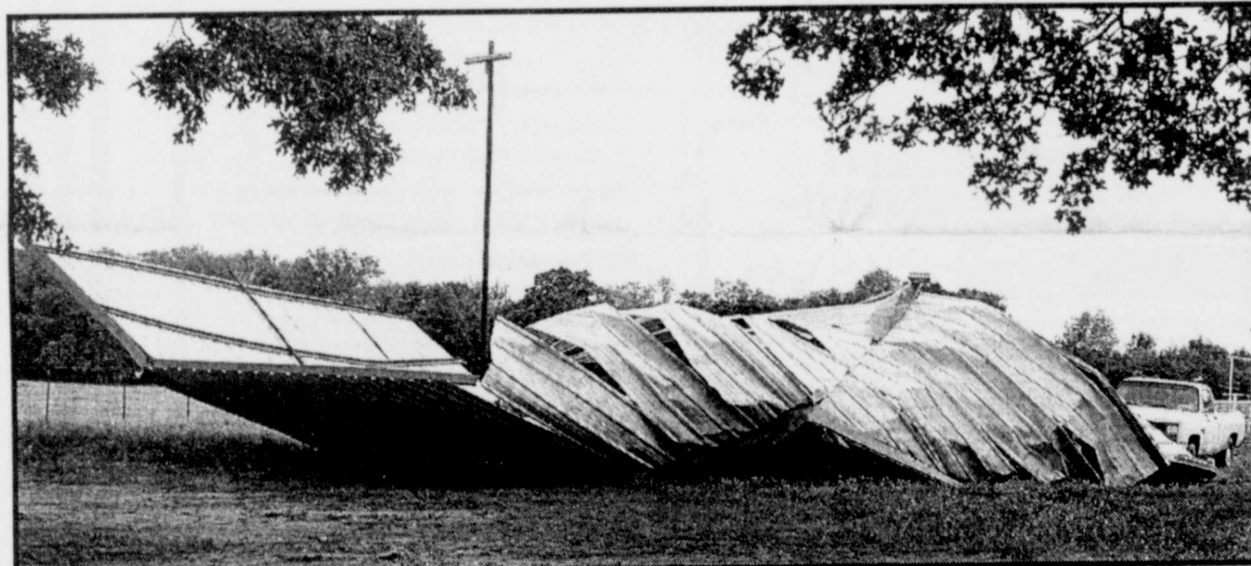
UPSIDE DOWN- High winds are responsible for destroying this equipment shed on Charles R. Davidson's property last Monday. Some reports of winds of up to 70 M.P.H. pounded buildings and trees in the Deport area.
