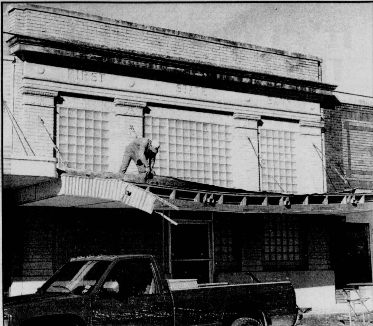
COMING DOWN -Guaranty Bank-Deport has recently been doing some work on the old bank building which they use for storage. The awning has come down, which does much to restore the building to it's original look. (Staff Photo)
