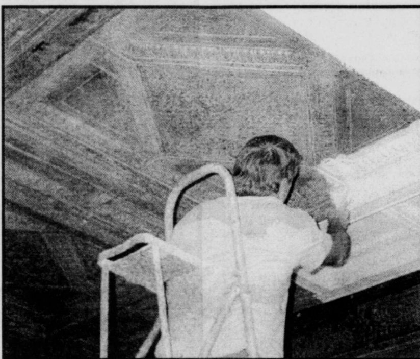
RESTORING the 100 year old tin ceiling in the old bank building at the south end of town is currently taking place. The building is newly remodeled and houses Relics, and antiques and collectibles shop plus an apartment. (Staff Photo by Mike Francies)
