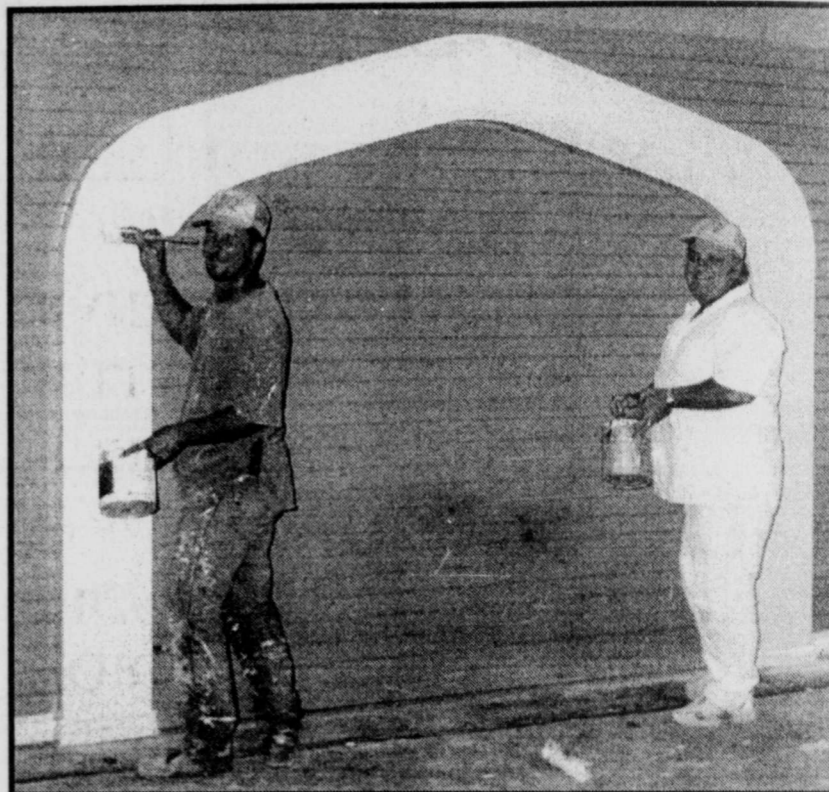
PAINTING the Chapel portion of Wood Funeral Home-Deport. Wood Funeral home is getting a total remodeling job to serve the community better. (Staff Photo by Mike Francies)
