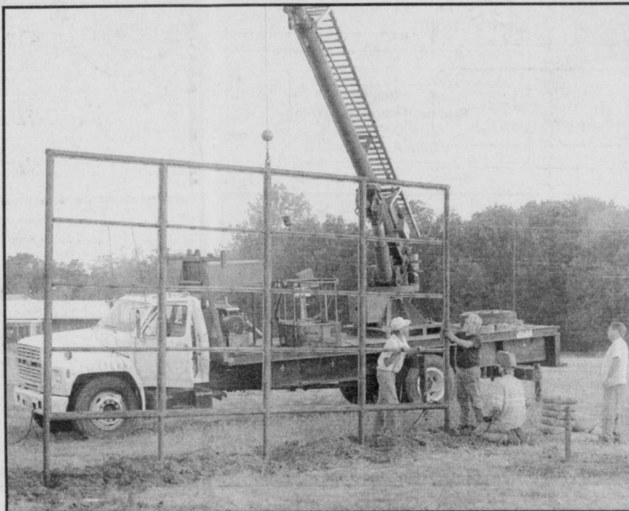
GOING UP -James Whitney, new resident to the Deport Area, helped erect the Downtown Deport sign which has been a project for the town recently. With the help of lots of volunteers, the sign will soon be completed with a big arrow pointing to downtown Deport, and will then have downtown businesses listed. (Staff Photo by Mike Francies)
