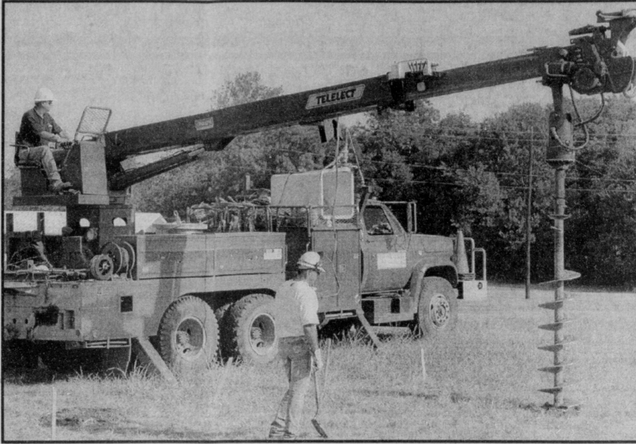
HOLE PROJECT -Texas New Mexico Power donated their labor to dig holes for the Downtown Deport sign which is being placed at the end of Main Street at Hwy. 271. (Staff Photo by Mike Francies)
