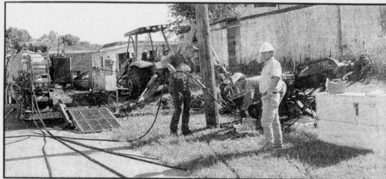
FIBER OPTIC CABLE is being installed from the GTE telephone facility in Deport to Bogata. Workmen were busy Tuesday on the project. (Staff Photo by Nanalee Nichols)
