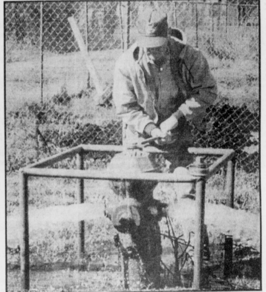
FLUSHING HYDRANTS -City water and sewer superintendent Herman LaRue sends water everywhere as the city of Deport flushed fire hydrants throughout town. The flushing helps clean water lines and makes sure that all fire hydrants are operational. (Staff Photo by Nanalee Nichols)
