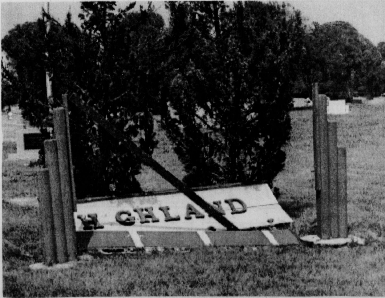
STORM DAMAGE-high winds last Thursday night completely destroyed the Highland Cemetery sign west of Deport. A fund raising effort is now underway to replace the sign with a metal sign similar to the "Welcome to Deport" signs on Hwy. 271. Anyone wishing to make a donation to this may do so by sending it to Highland Cemetery Assn., P.O. Box 334, Deport, TX. 75435 (Staff Photo by Thomas Nichols)
