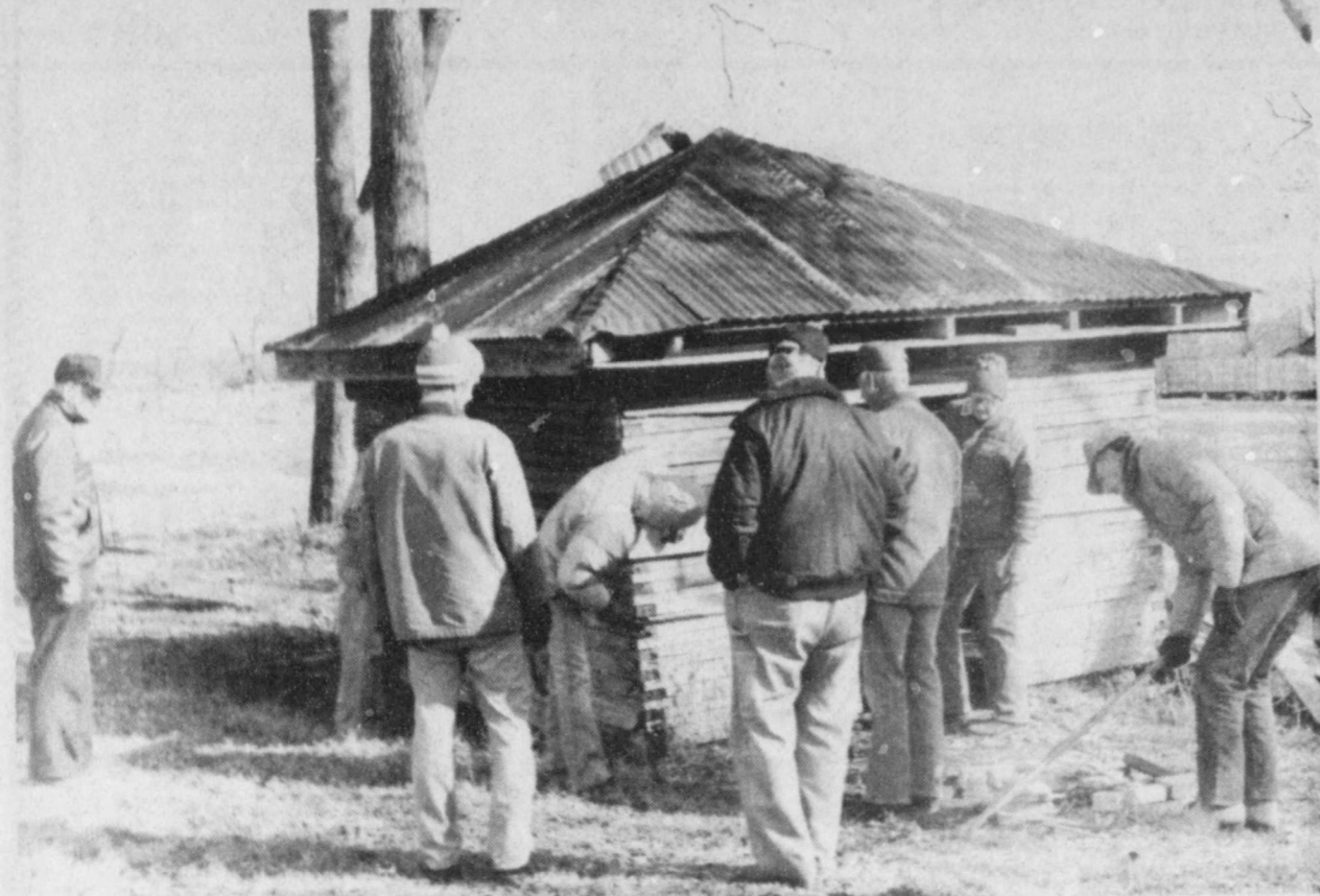
THE DEPORT KIWANIS Club worked on bracing the old Deport Jail last Saturday morning. The club plans to move the jail to its new concrete foundation for re-storing as soon as weather permits. (Staff Photo by Thomas Nichols)
