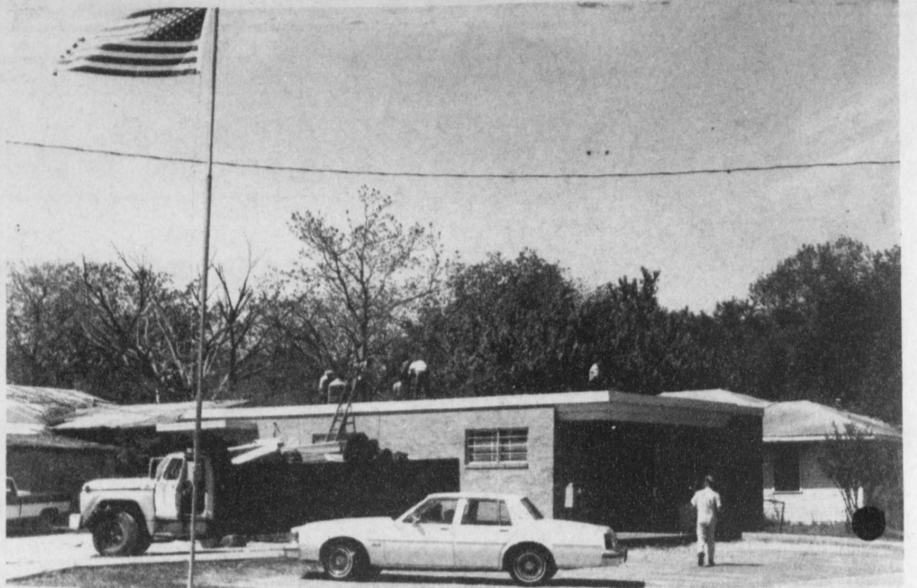
NEW ROOF-The Deport Post Office has been receiving a new roof this past week. In spite of hot
