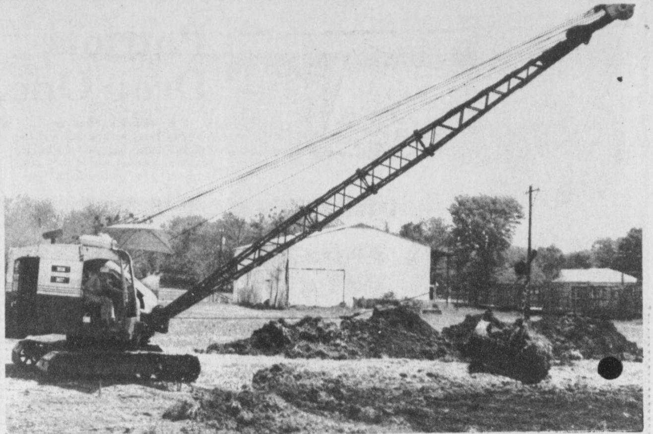
DIGGING AWAY -A dragline is dredging the creek where it runs through Deport to provide better water flow. The new bridge at the
