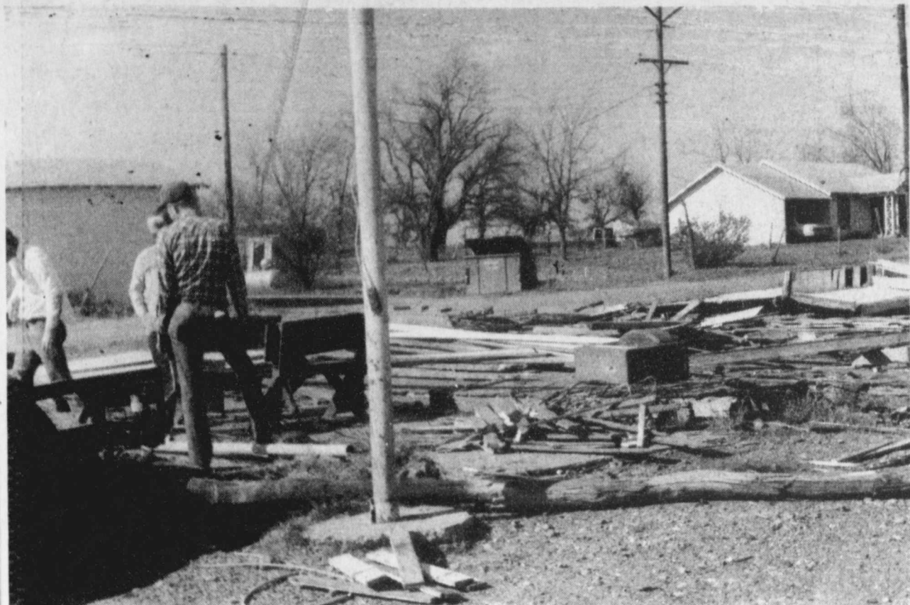
GONE -The old Pattonville Grocery has been torn down, and will be replaced by a new structure soon. Glen Biddle will build the new structure and operate it. (Staff Photo)
