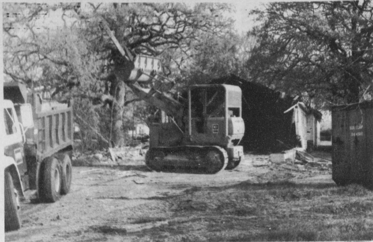
GOING, going gone. The old bus shed at Deport Elementary School campus was bulldozed to the
